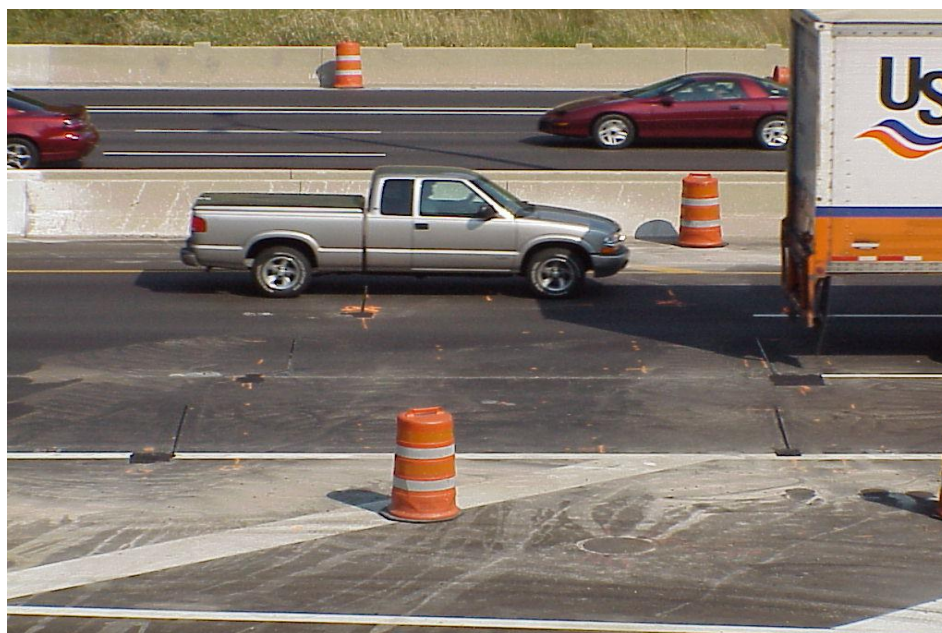
FIGURE 4.3. Pavement-embedded detectors, saw cuts and pull box visible.
