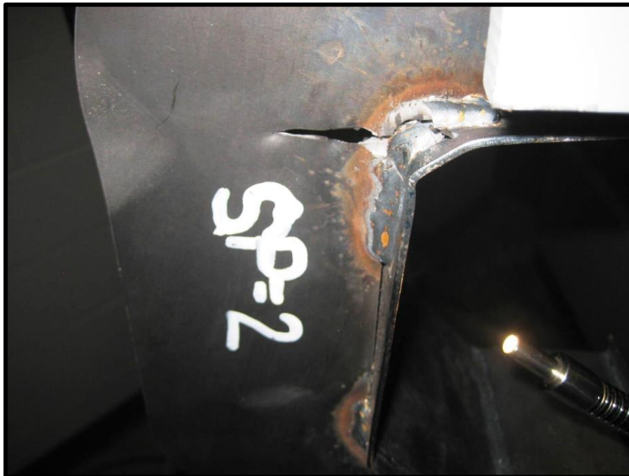
Figure A3. Photo of the end of test for Specimen 2.
