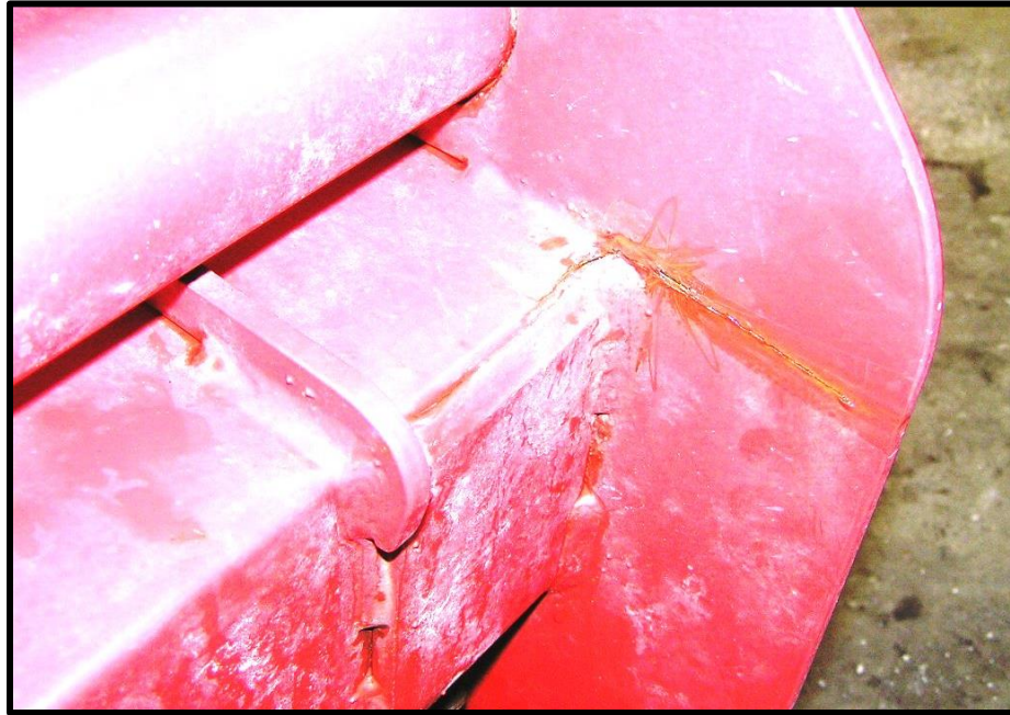
Figure D3. View of a typical field failure (inner surface of rib)
