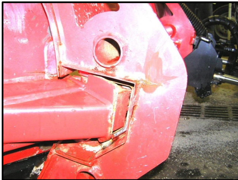
Figure D2. View of a typical field failure (outer surface of rib)
