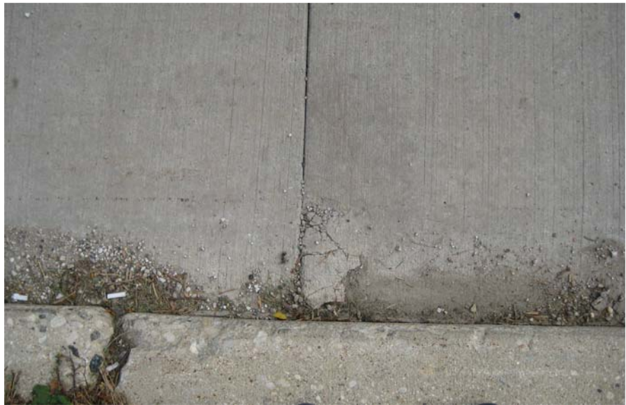
Figure 3.4: 87 th Street Bus Pad Test Section, Corner Spall Near Curbline
